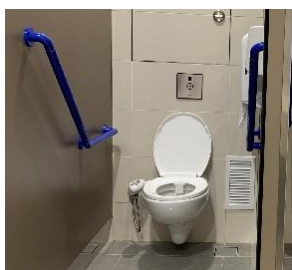
Ambulant disabled toilets
